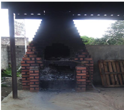
Figure 2: Incinerator at Mulenga Clinic in Kitwe
